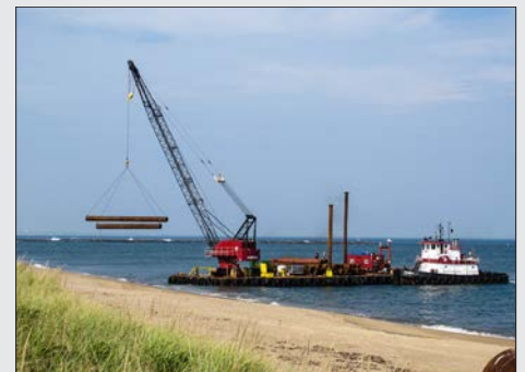
GZA coordinated dredging activities with the USACE, municipalities and regulators to permit the beneficial use of dredge materials for this beach nourishment project
