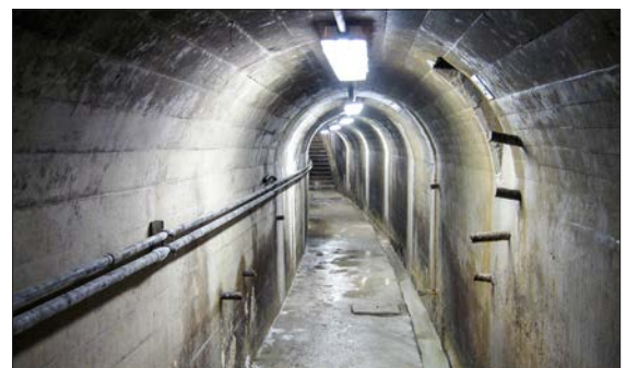
As part of its Dam and Levee inspection services, GZA performs inspections, drilling and instrumentation installations in structures such as this inspection galley located deep within a concrete gravity dam
