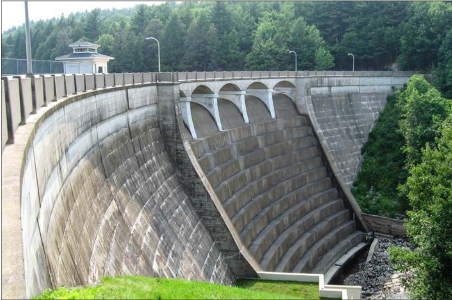
GZA performs subsurface investigations; above- and below-water visual and rope-access inspections; and hydrologic & hydraulic, stability and seepage analyses on government dams throughout the United States
