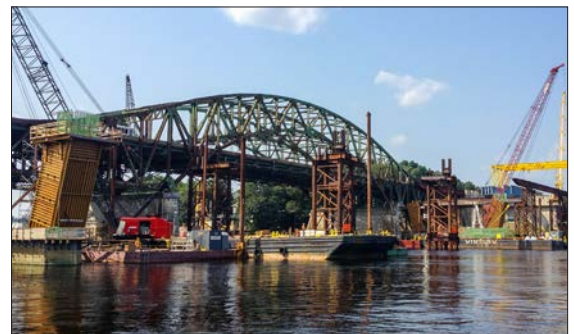
Geotechnical and structural design services for temporary steel sheet cofferdams, precast bridge pier walls and support of excavation of bridge abutments
