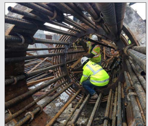
GZA engineers installing instrumentation in a drilled shaft cage in preparation for thermal integrity profile (TIP) testing
