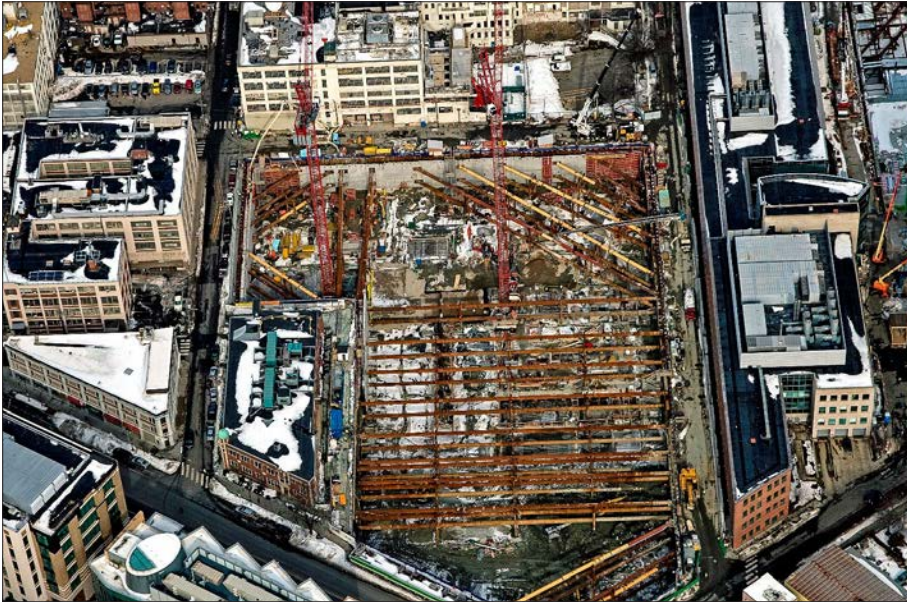
Geotechnical and structural design services for temporary support of excavation in a 45-foot-deep cut
